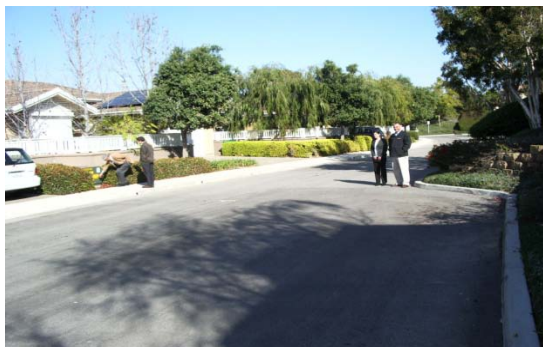
Block #1 of the four blocks of faculty homes for the zero net energy (ZNE) home sub-project at the University of California Irvine. On the left side of the road are Jerry Thode and Gordy Stecklein of SCE. They are near the pad mounted transformer that feeds the eight homes that will have the maximum retrofit to become ZNE. On the right side of the road are Christina Haddad of EPRI and Dar Mardan of SCE. They are near the location where the community energy storage (CES) battery system will be installed.
