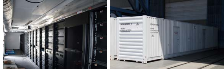
Figure 8: Inside and Outside of SCE's Containerized 2MW lithium-ion Battery to be located on a 12kV circuit primarily used with dispatching DER
