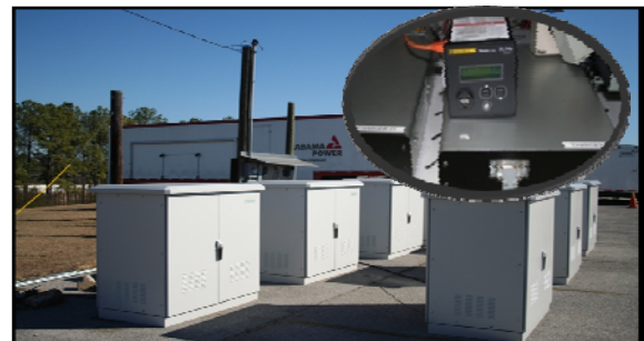
Figure 6: Battery Units with Ion 7330 Meters
